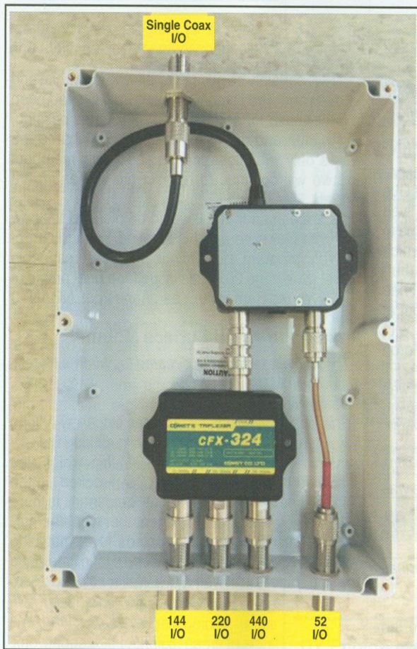
Photo C. Weatherproof housing at base of four-antenna mast. Note this is an early picture. The top connector has since been moved to the bottom to prevent moisture potential — though that has not been an issue recently in light of California's severe drought.
